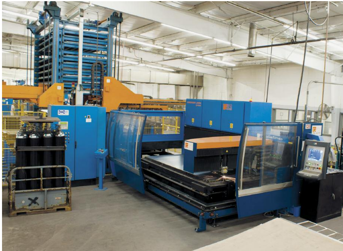
In order to expand its laser cutting capabilities, Pulverman purchased a Prima Platino 2D laser system with a 10-shelf TowerServer in 2004. The Platino is equipped with lasers developed and produced at Prima Industrie in laser powers ranging from 3000 to 5000W. The laser cuts a broad range of materials and thicknesses with speed and precision without the need for manual adjustments.
